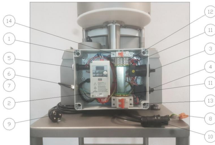
Figure 17. Electrical cabinet overview
